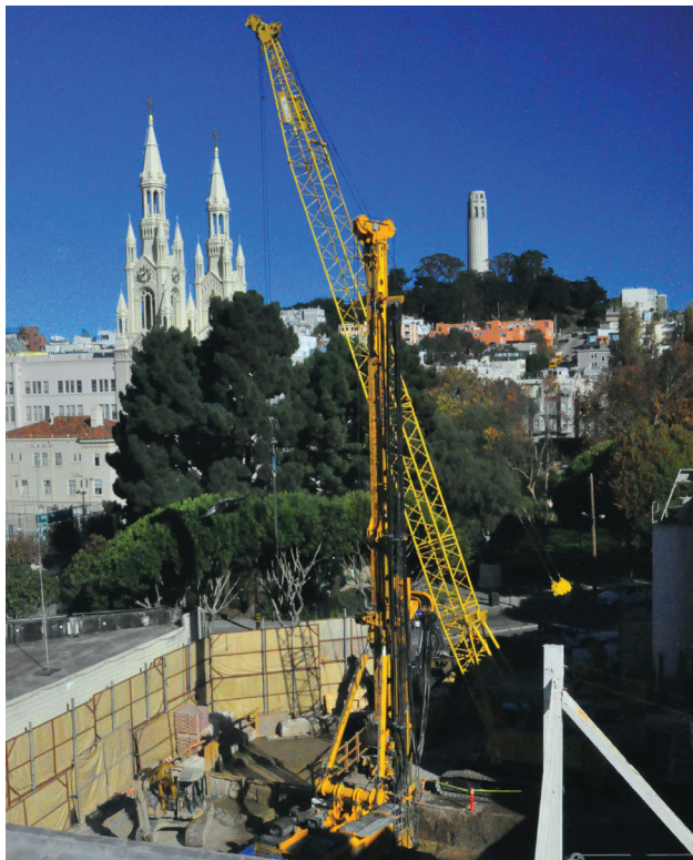
Pagoda site (foreground) facing Washington Square Park and Coit Tower. Construction abuts historic buildings and parks, and may continue for up to 6 years or more.
