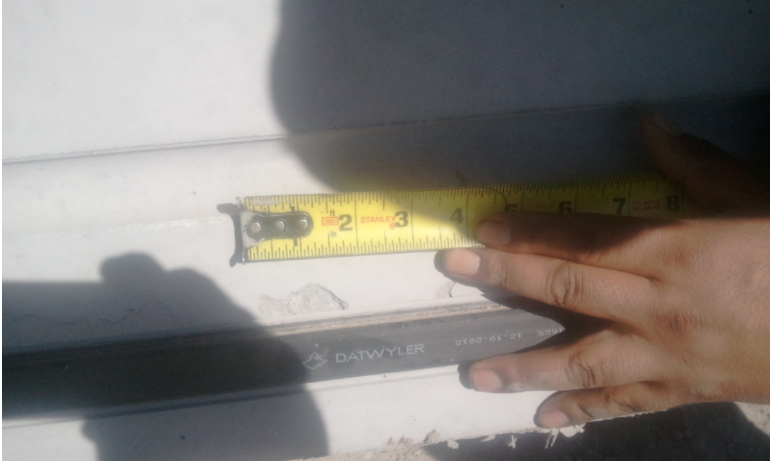
Photo 2. Spall on the radial joint near the footed gasket
