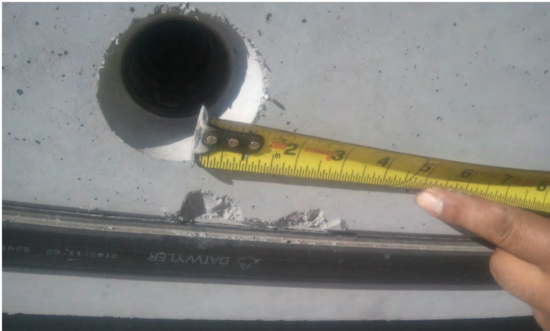
Photo 3. Spall on the circumferential joint near the footed gasket
