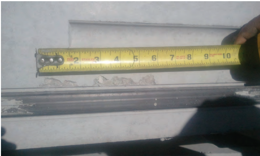
Photo 1. Spall on the radial joint near the footed gasket
