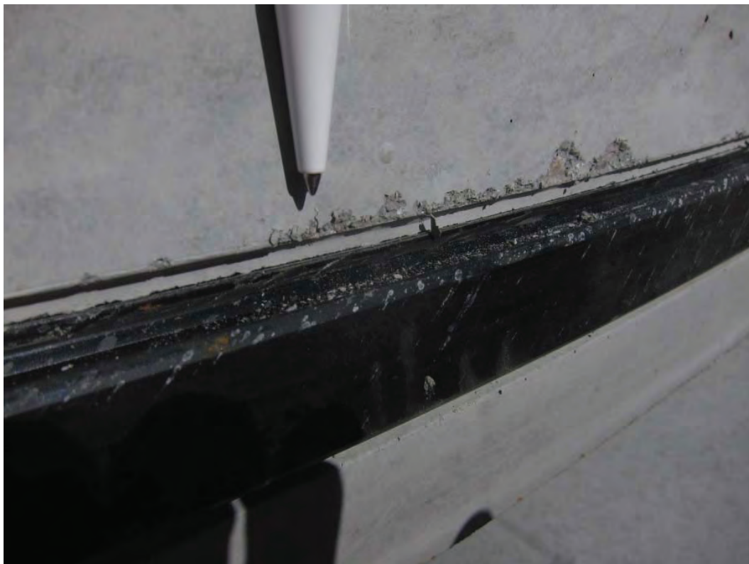
Photo 2. Close-up of spalling along the circumferential face above the gasket area. Note spalling height \sim 3/8 " and spalling length \sim 8 "
