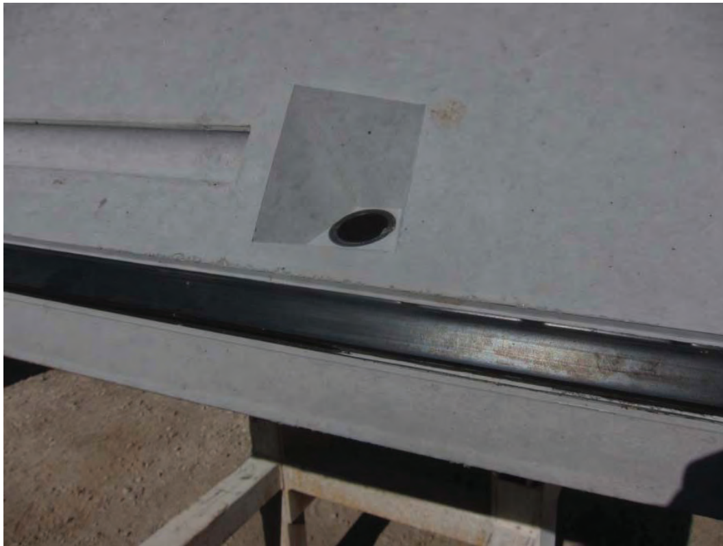
Photo 1. Spalling along the circumferential face above the gasket area
