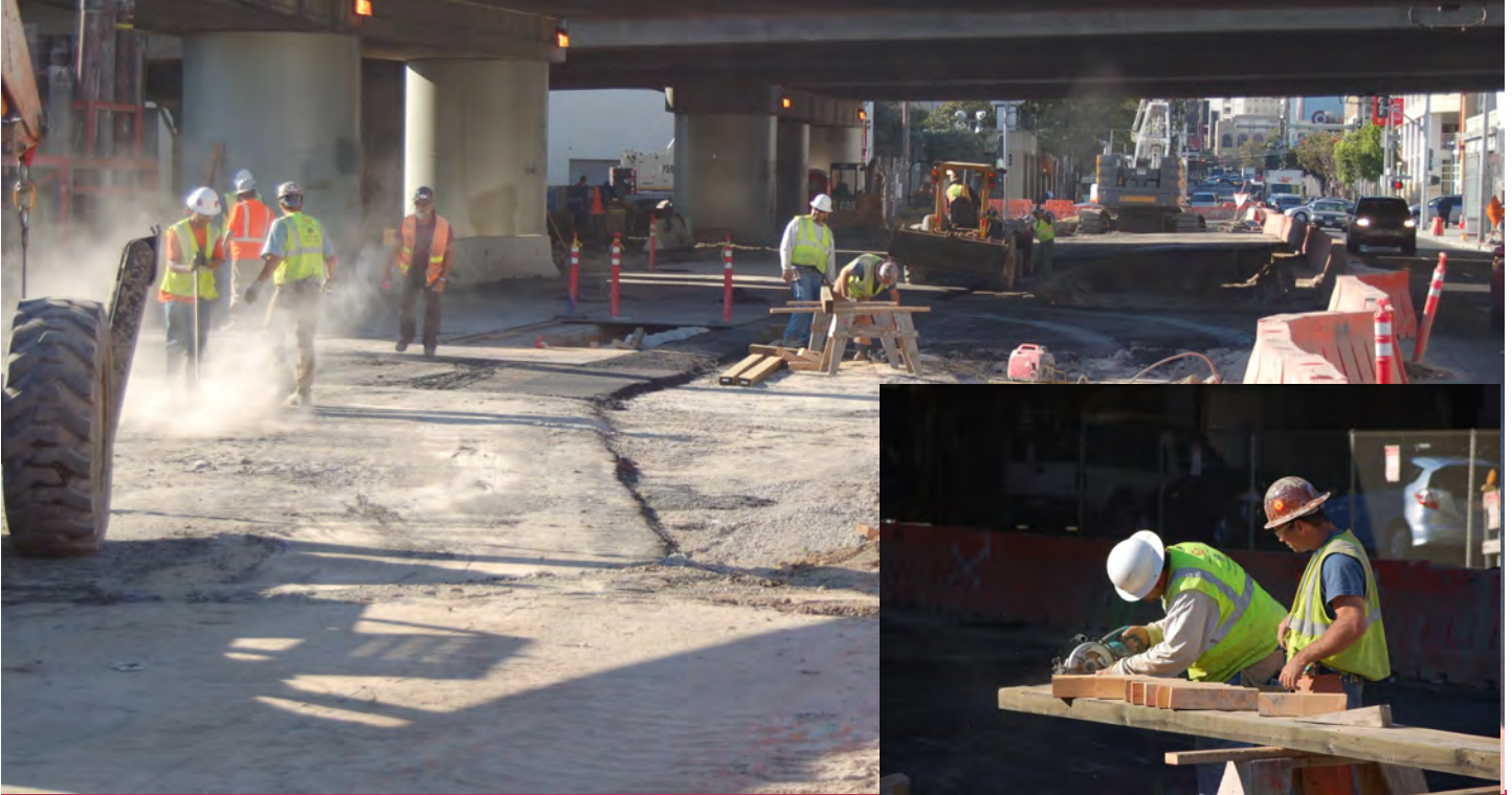
Slurry wall preparation work on at the TBM launch site under Hwy. 80.
