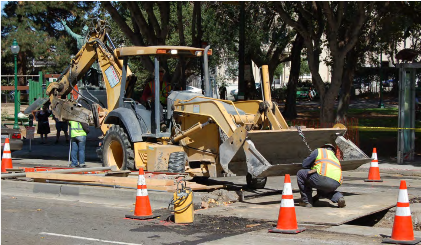
Utility relocation work in North Beach uses steel road decking panels when work is completed each day so traffic can flow through the work site during peak hours and local businesses and their customers have normal access.
