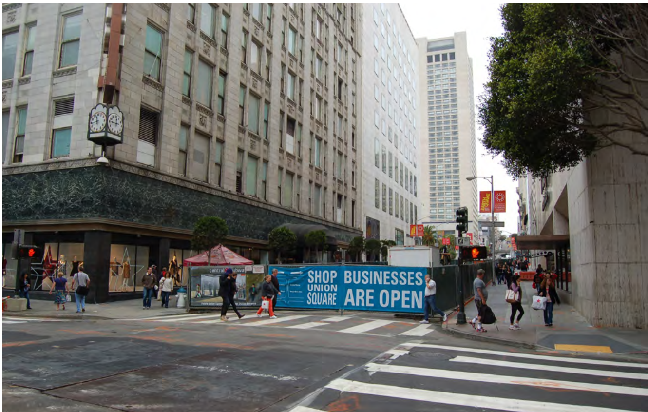
New banners guide and inform shoppers and tourists that local Businesses Are Open next to full-scale construction.
