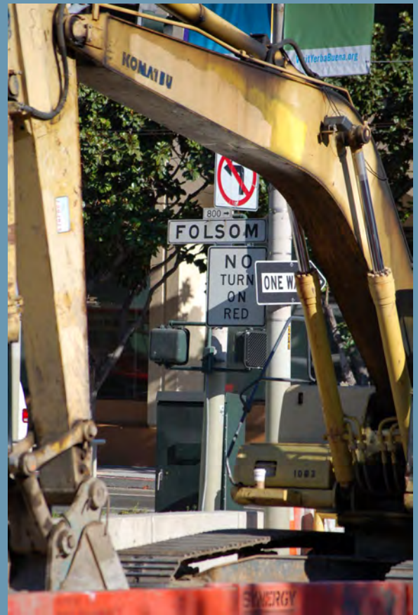
The Yerba Buena/Moscone Station will be constructed at 4th and Folsom streets.
