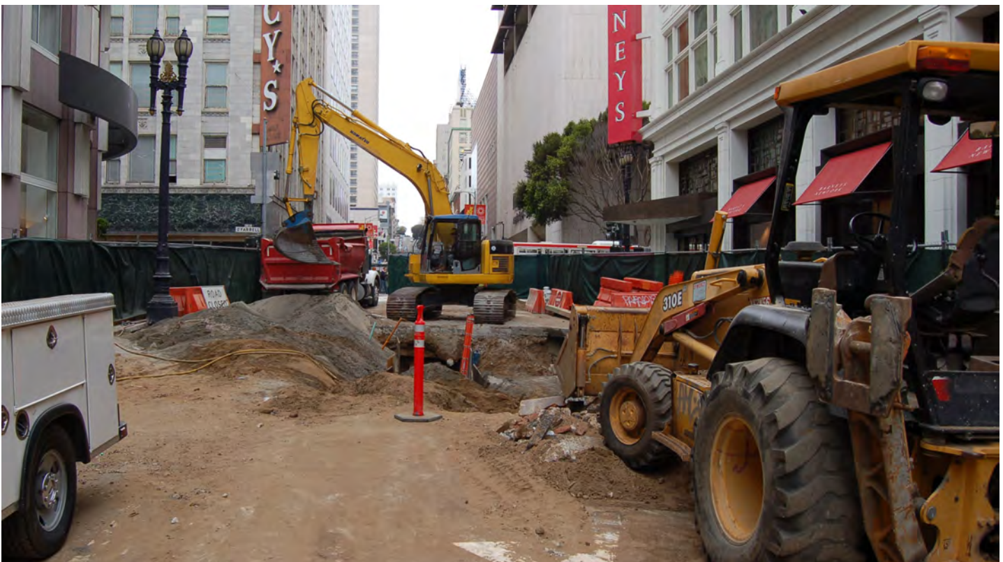
On Stockton Street looking north to O'Farrell, demolition of the now obsolete utility infrastructure is underway at the future Union Square/Market Street Station headwall installation, ahead of the upcoming holiday moratorium.
