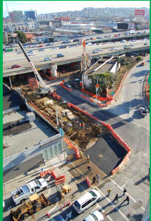
The tunnel launch box site, as seen from the roof of a Whole Foods building.
