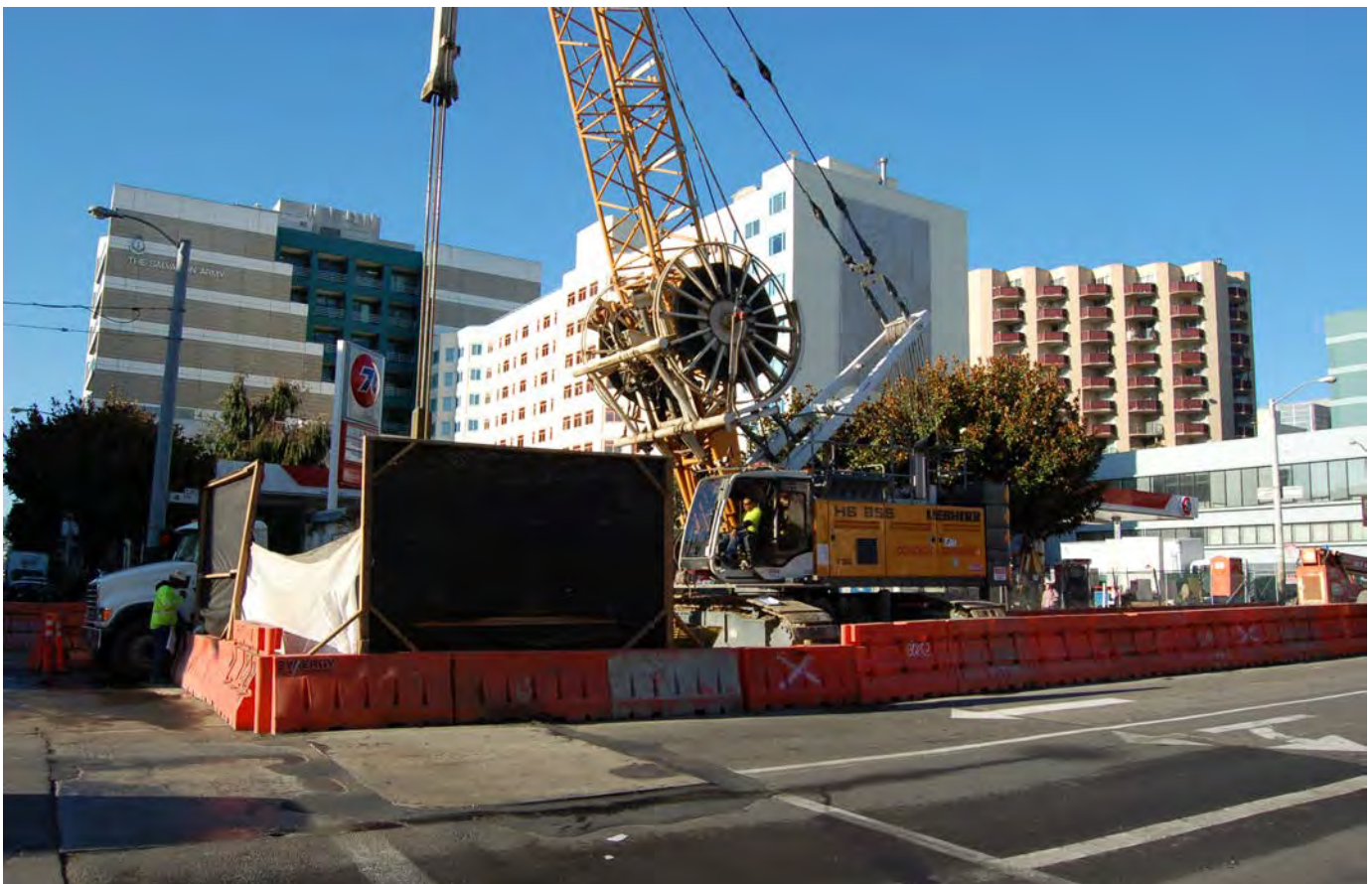
This is a picture of the excavation operation at the South Headwall at Moscone/ Yerba Buena Station.
