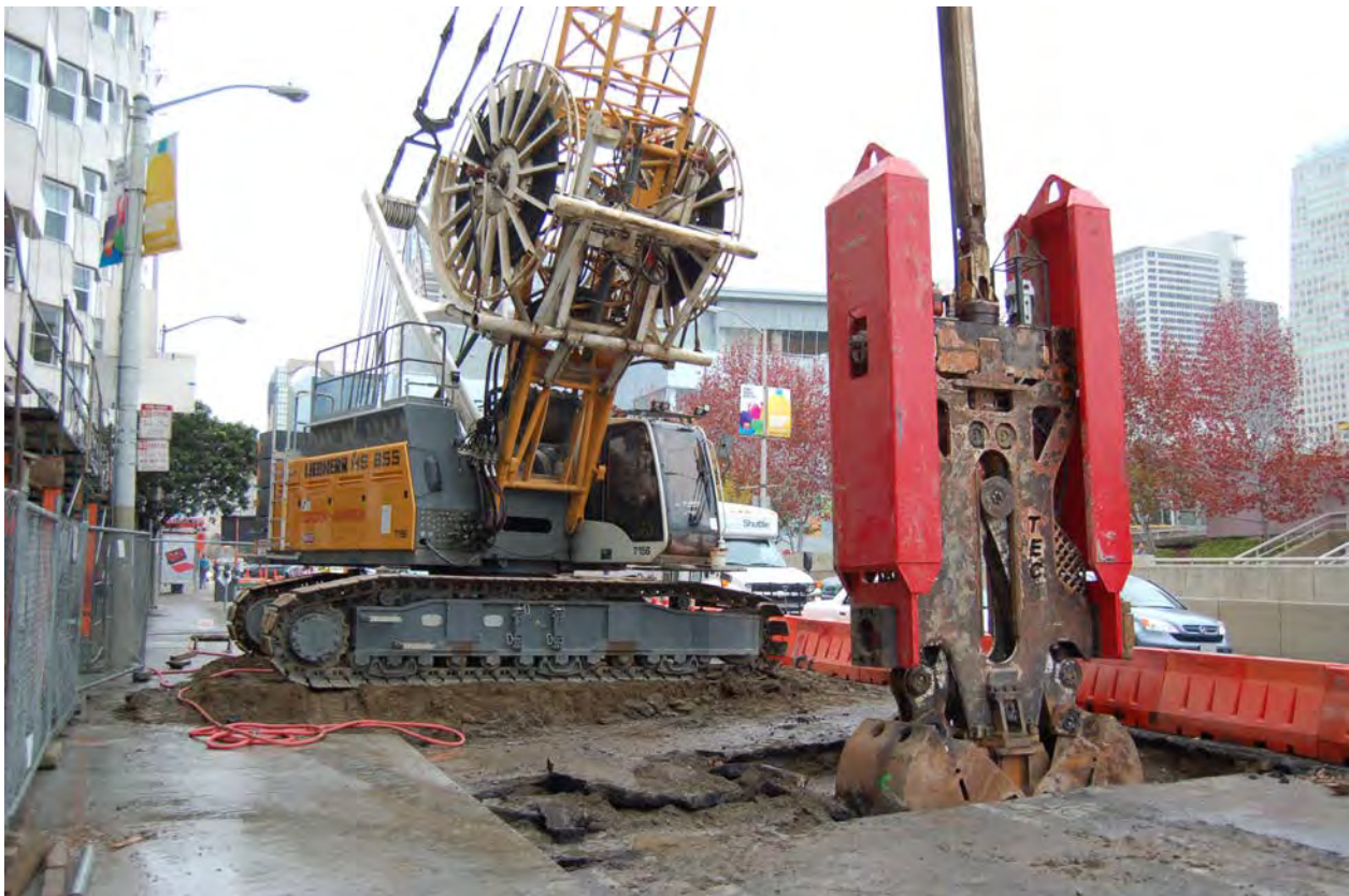
This is the construction site at the Moscone/Yerba Buena Station. Currently the CN1252 contractor is digging out the locations for the the Moscone Headwalls which fall under the Tunnel Contract.
