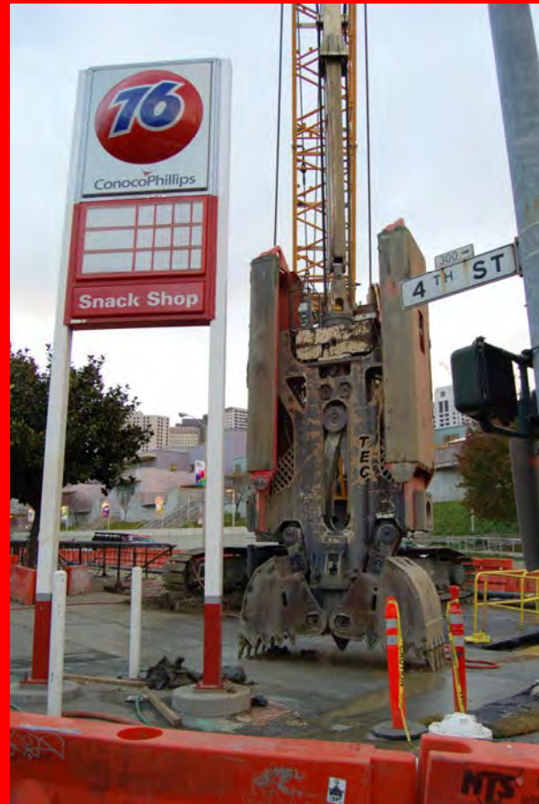
Slurry Wall excavation equipment used for the Headwalls at Yerba Buena /Moscone Station.
