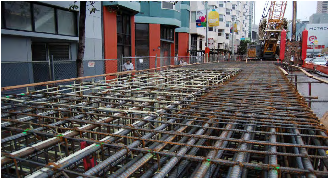
Fabrication of the rebar cages for the Headwalls at Moscone/ Yerba Buena Station. These cages will be lowered into the slurry filled pits. Then after the rebar cages are in place the pits will be filled with concrete as the slurry is pumped out of the excavated holes.
