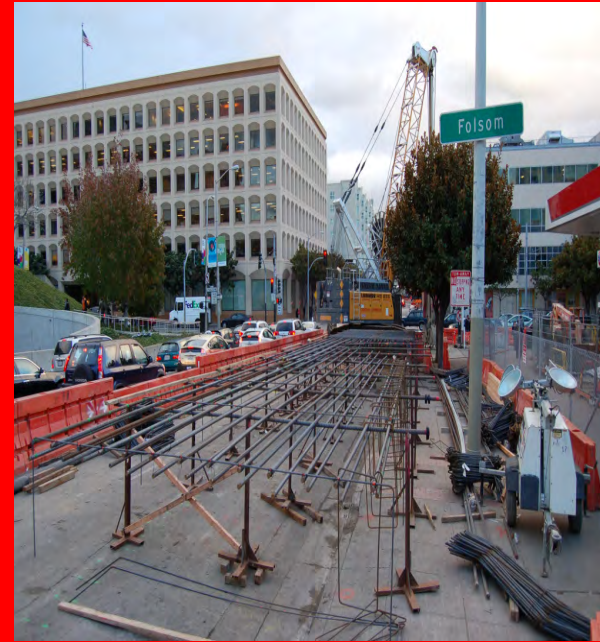
Reinforcing Steel for Slurry Wall panel at Yerba Buena /Moscone (YBM) Station Headwalls.
