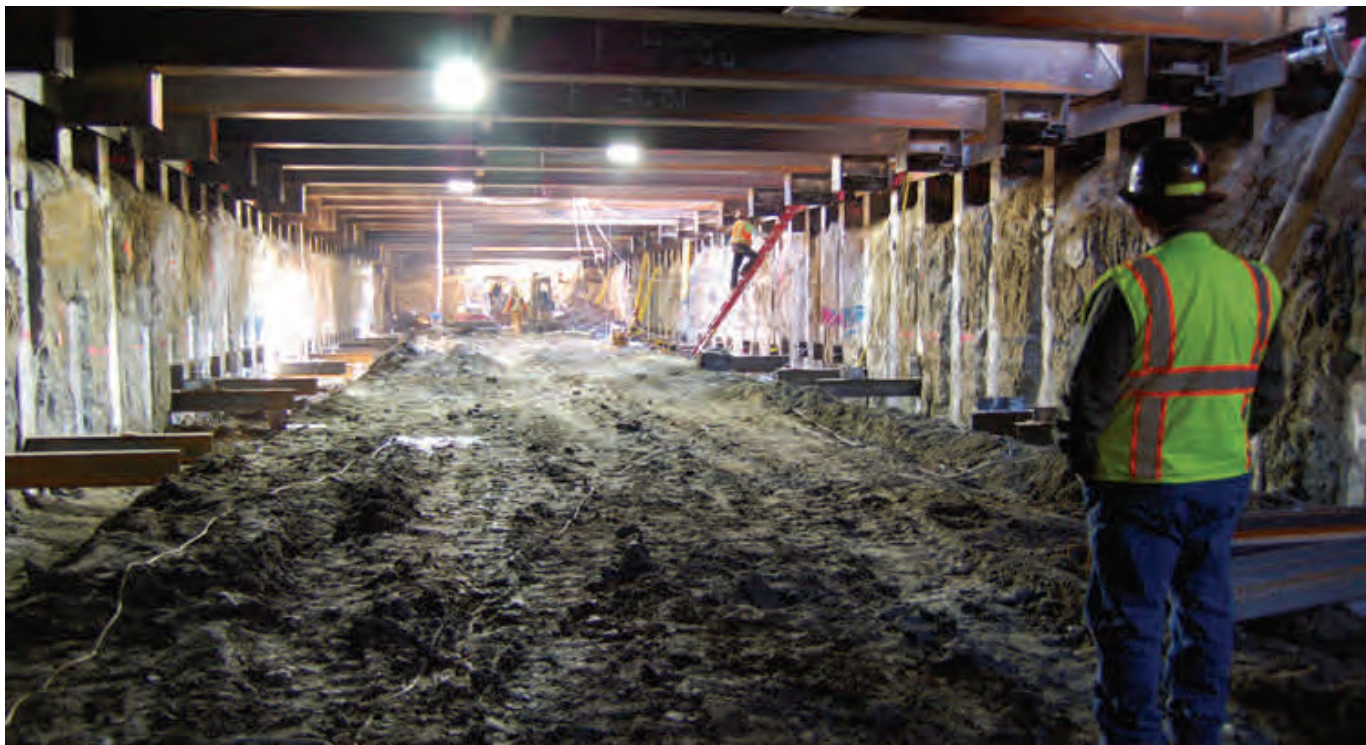
A safety inspector surveys the launch box site at 4th Street in SoMa. Excavation work is ongoing and bracing is installed as material is removed.
