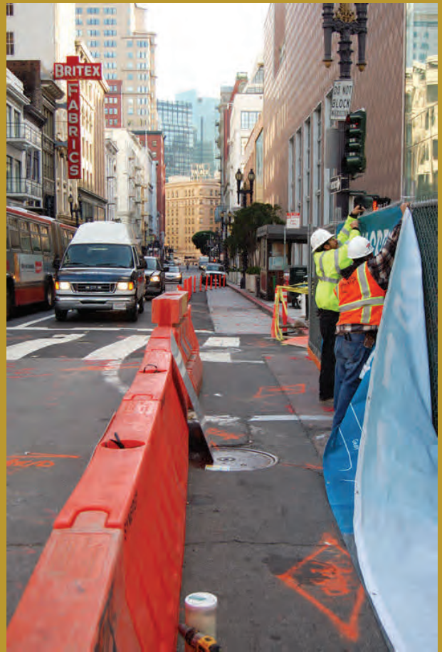
Workers re-install Central Subway project banners following the end of the 2012 holiday moratorium
