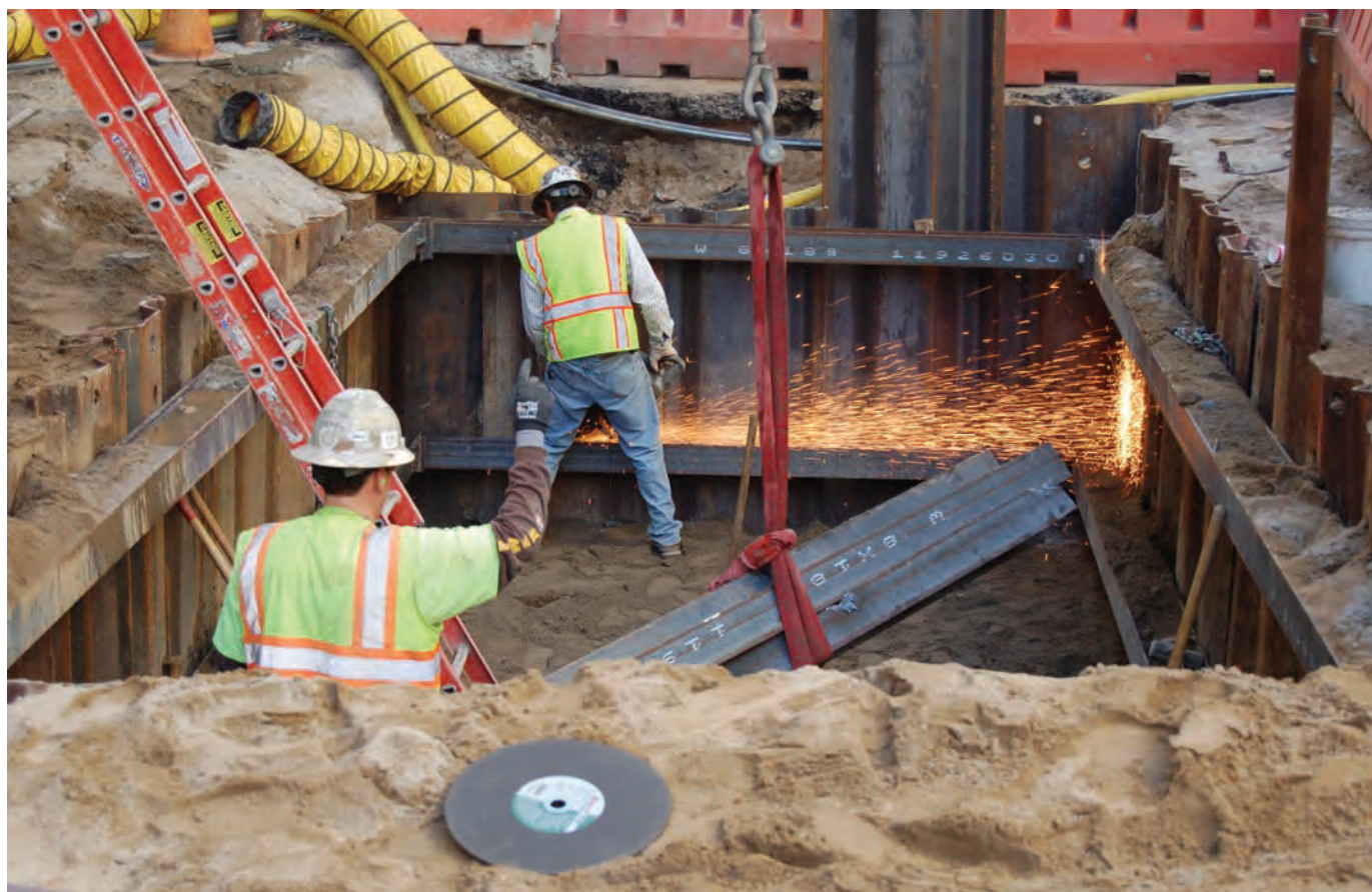
Workers remove bracing from an excavation being backfilled at the Union Square/Market Street station site.
