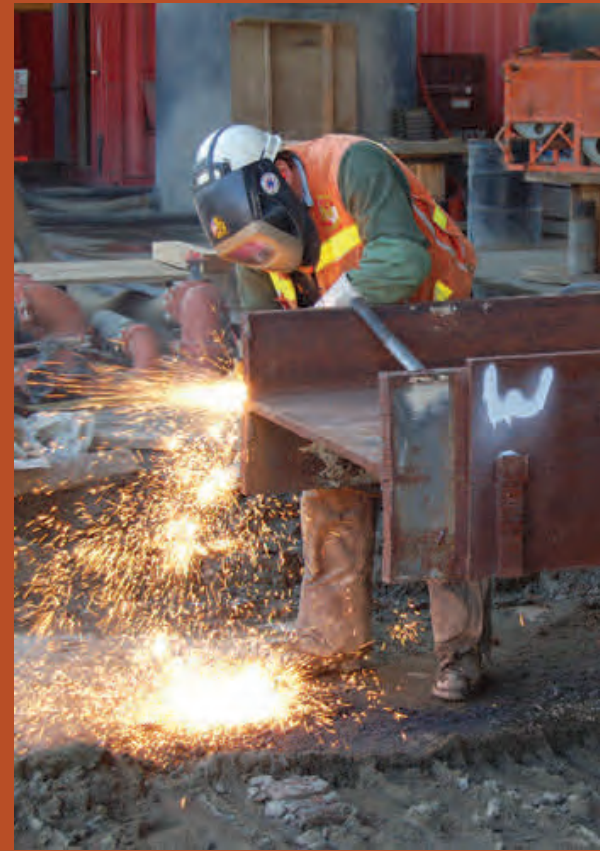
A welder works on bracing that will be used to support the walls of the launch box on 4th St.
