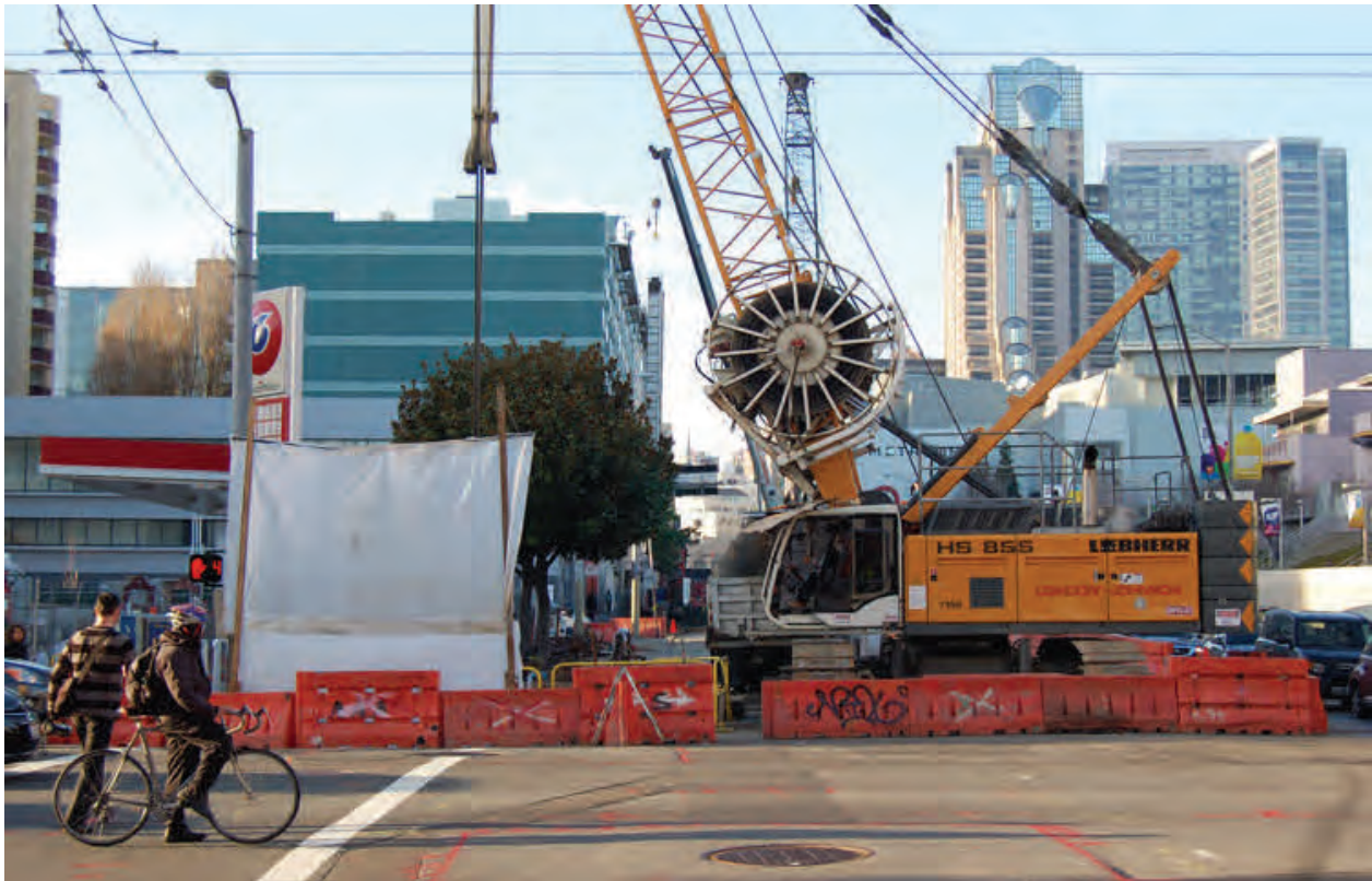
Crews use a crane and clamshell digger to excavate the future Yerba Buena/Moscone station headwalls, ahead of actual station construction which will take place under Contract 1300. The station entrance will be located on the site of the 76 gas station pictured here, photo left.
