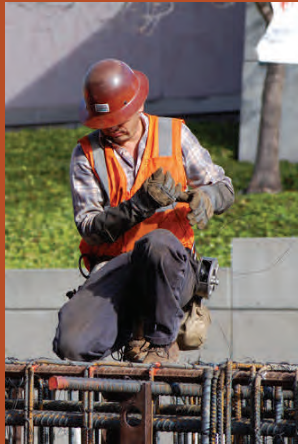
Several giant rebar cages have been lowered into deep shafts to provide structural support at the Yerba Buena/Moscone station headwalls.
