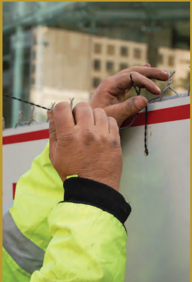
A worker uses steel wire to firmly install construction site safety signage.
