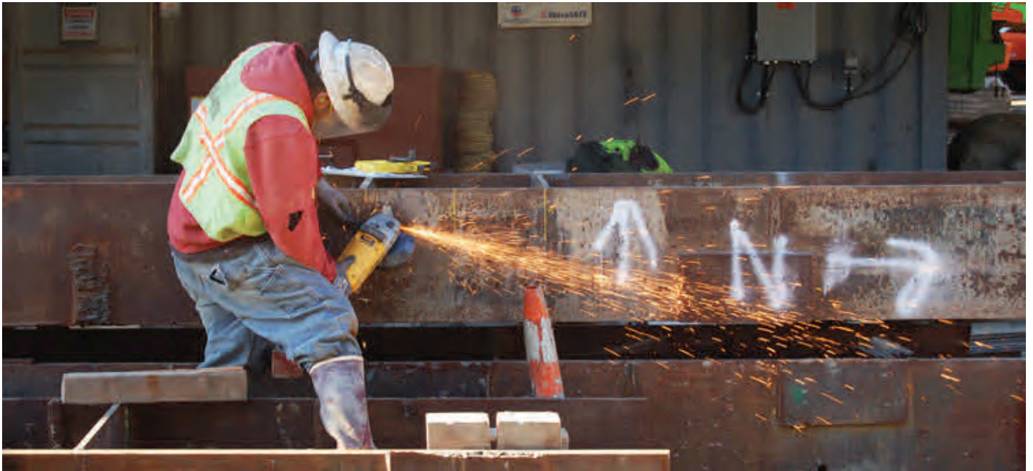
A worker prepares the surface of a steel I-beam which will be used to brace the walls of the 4th Street launch box.
