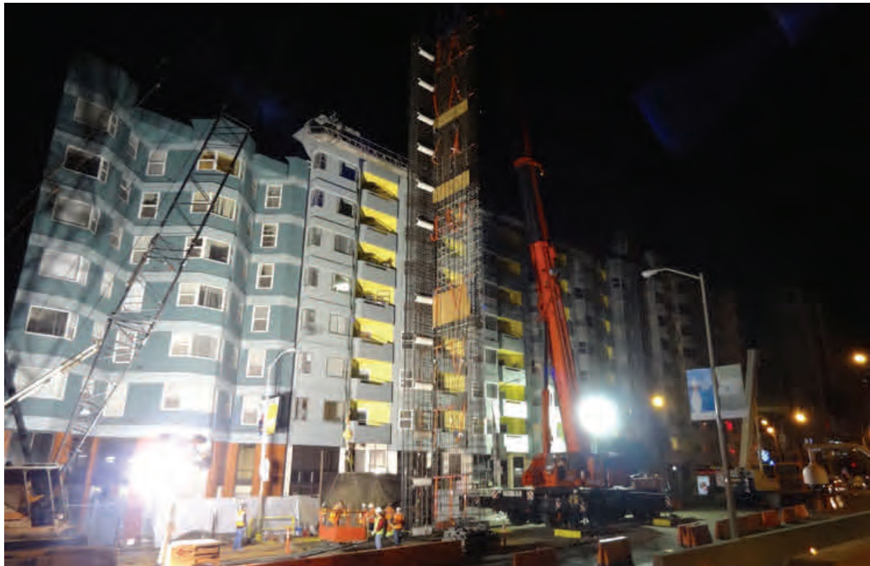
Crews at the future Yerba Buena/Moscone station site lower one of many rebar cages into place prior to pouring concrete for the station headwalls.
