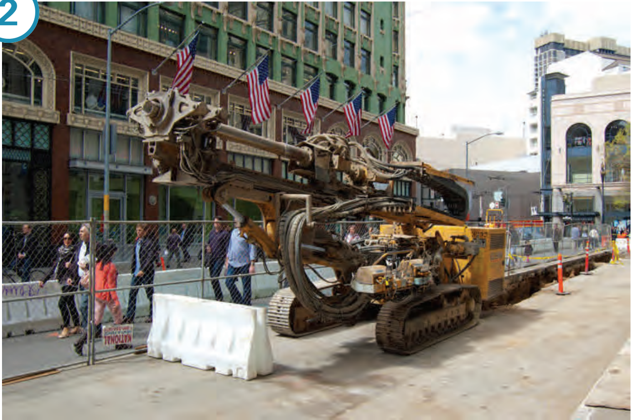
4th Street between Market and Stevenson, where preparation for compensation grouting will soon begin.
