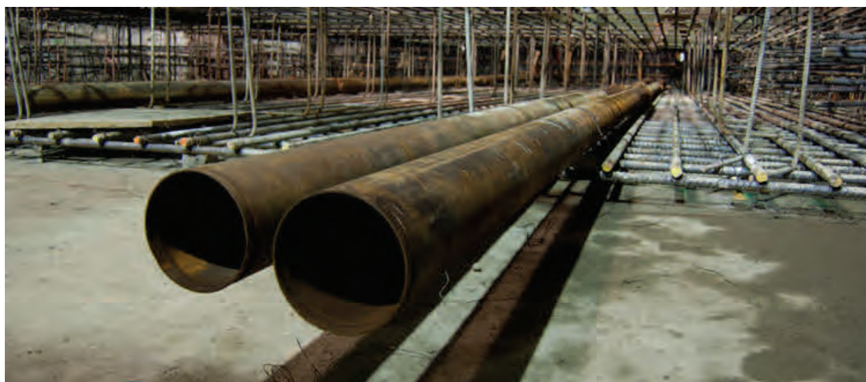
A close-up of piping and rebar that will reinforce the launch box floor slab.
