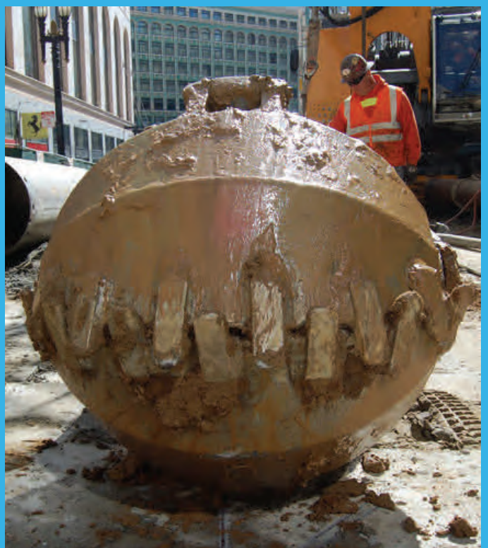
Below - A close-up of the clamshell bucket excavator used to dig the secant pile shafts used in the southern Union Square/Market Street Station headwalls.
