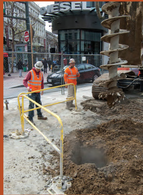
Workers performing drilling operations head of building the large vertical shaft at the corner of Ellis and Stockton.
