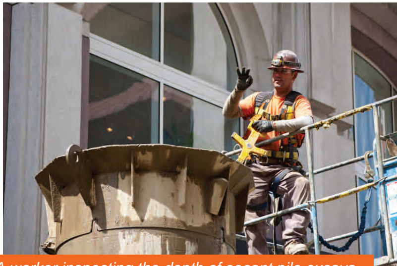
A worker inspecting the depth of secant pile excavation for the Union Square/Market Street headwalls.
