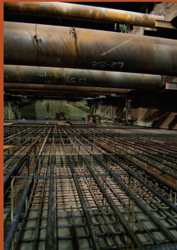
Looking north in the TBM launch box, with temporary supports above, and rebar for the future floor slab below.
