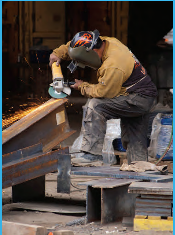
Above - A worker uses a grinder while fabricating temporary supports that will be used to shore up the launch box before the floor slab is poured.
