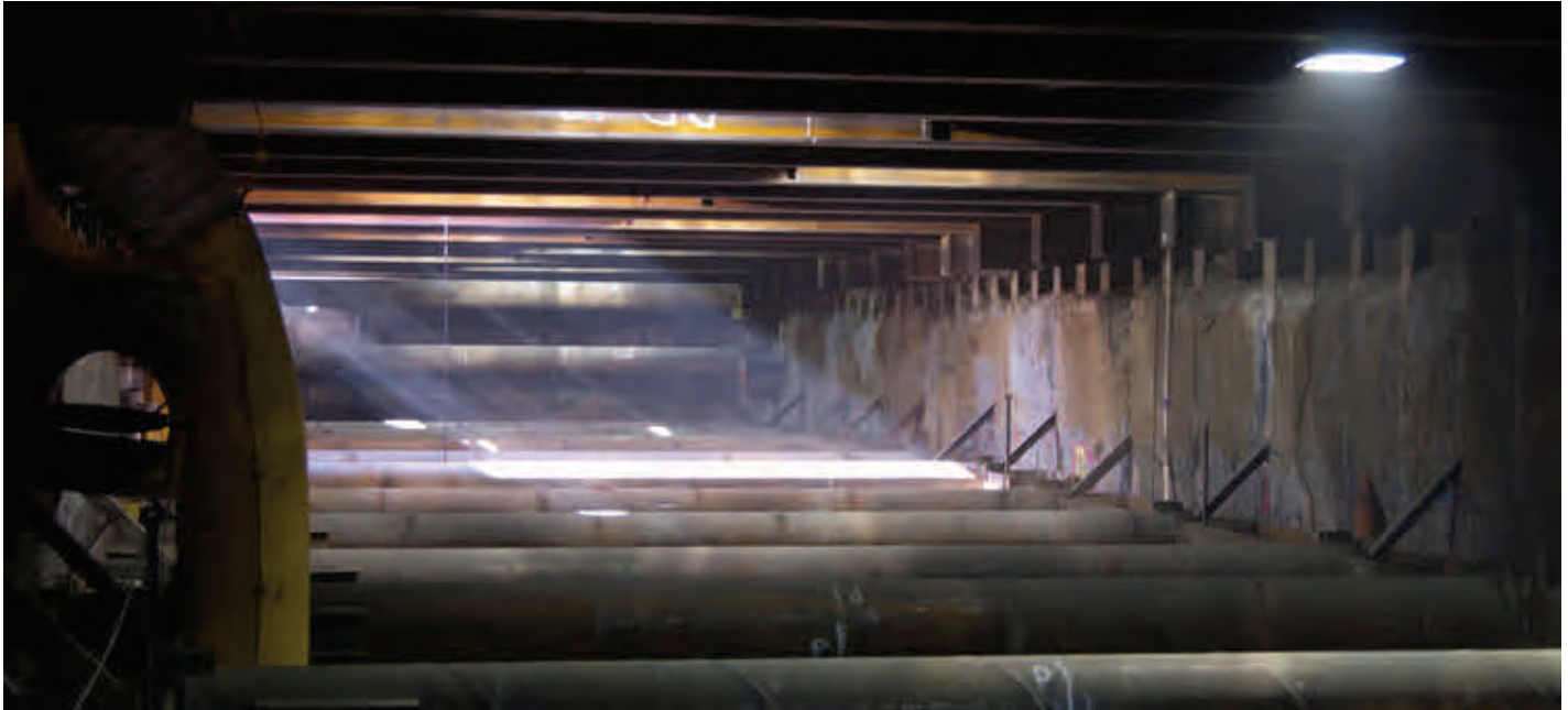
View looking north at the tunnel boring machine launch box site, showing temporary supports in place.
