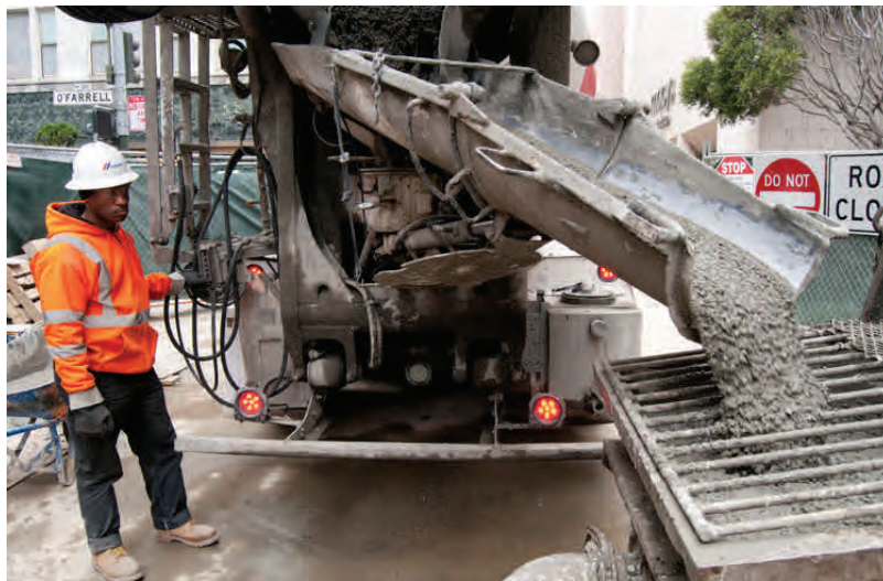
Concrete pour for Union Square/Market Street station headwall pile, south of O'Farrell.
