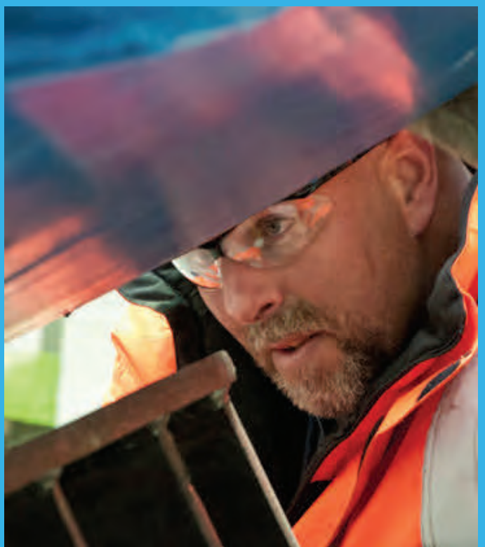
Below - A worker monitors the lowering of ring 1 of the TBM Mom Chung. Precision is paramount, and final distances were measured in millimeters.
