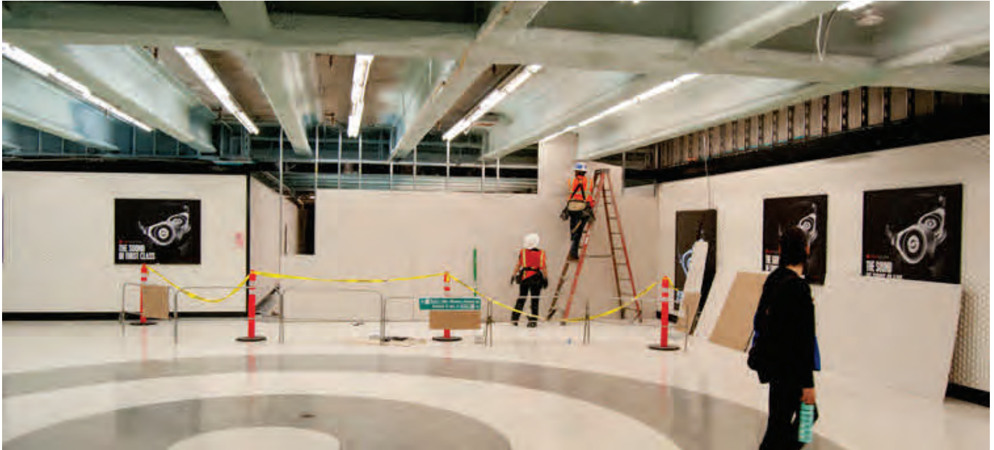
A view of the temporary wall going up in the Powell Street subway station.
