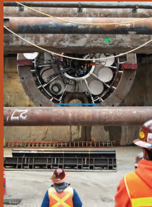
Workers monitor progress the TBM Mom Chung is lowered into place at the launch box ramp.
