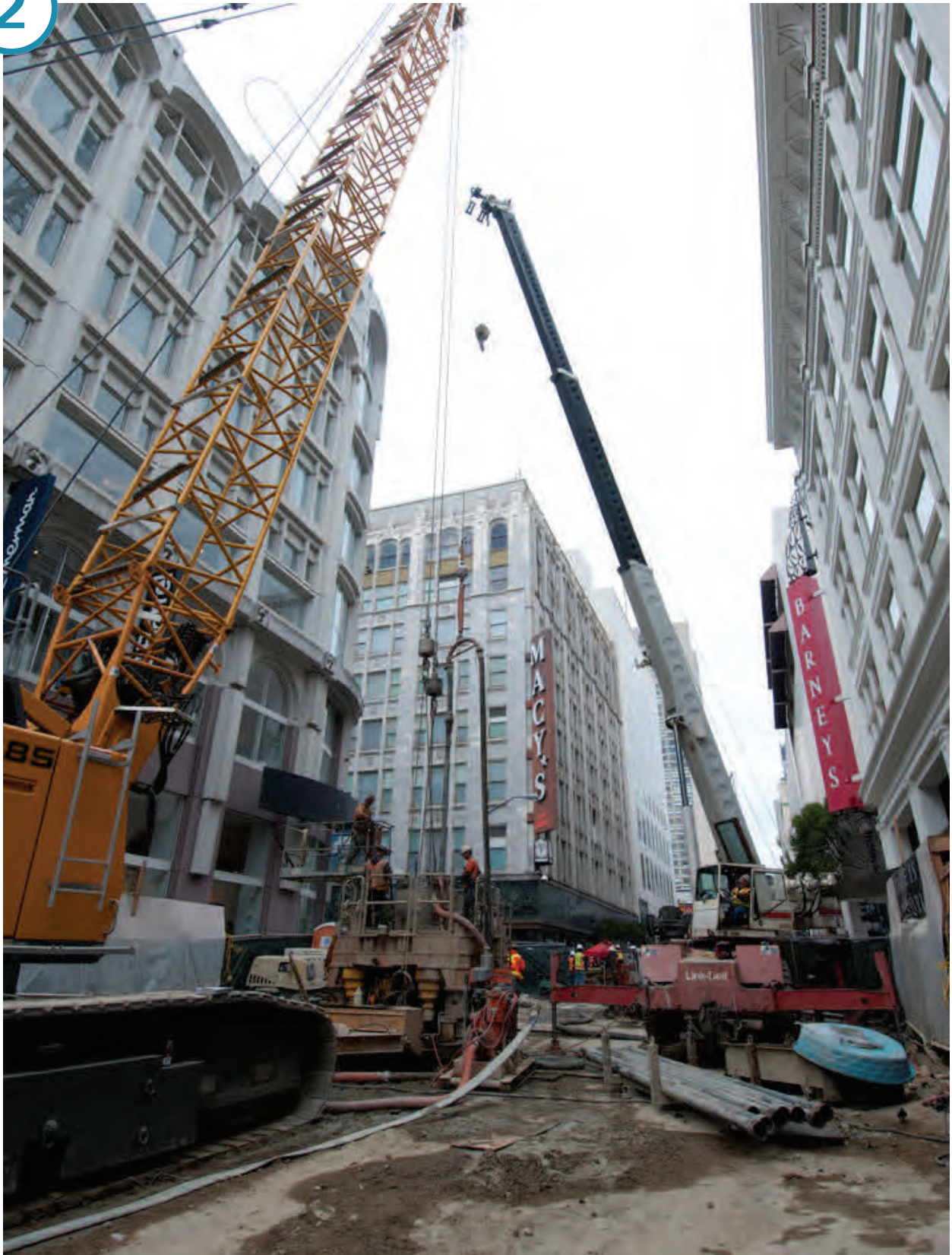
Looking north up Stockton Street, toward O'Farrell. Crews are excavating interlocking, subsurface shafts that will form the headwalls of the future Union Square/Market Street Station.
