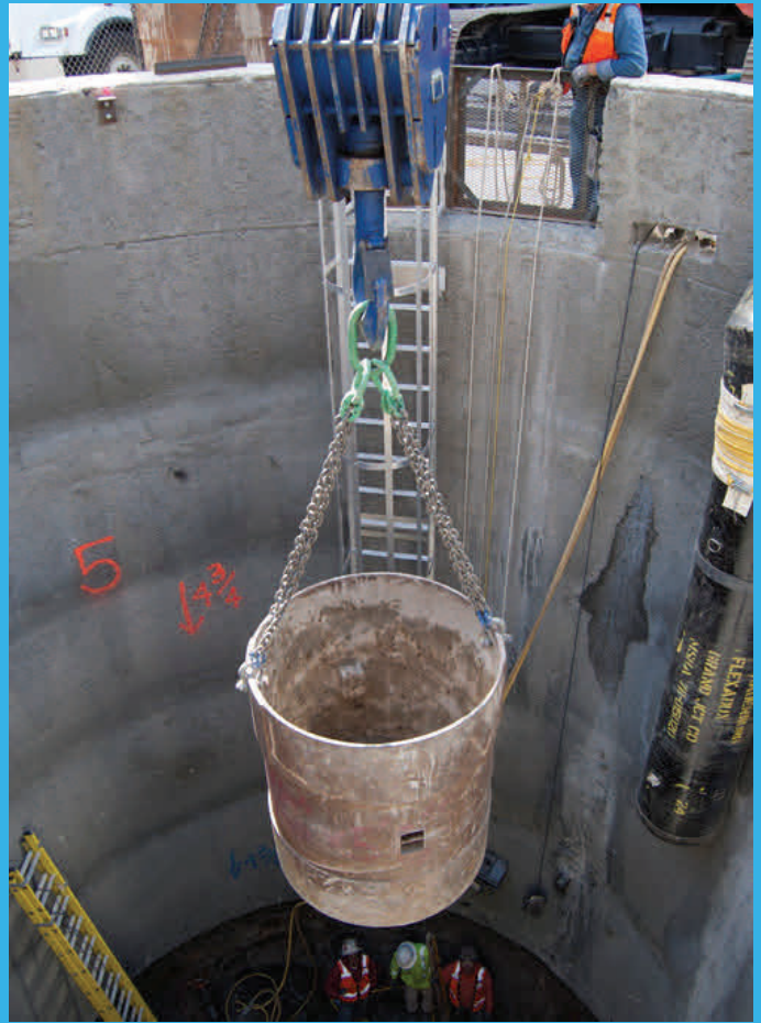
Above - Crews use a large steel bucket to remove spoils excavated from the large-diameter shaft currently being excavated at Ellis and Stockton.
