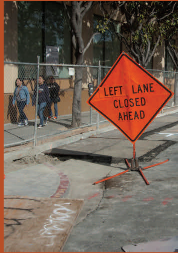
Work is near an interim completion stage on 4th Street between Folsom and Harrison, installing subsurface piping used in compensation grouting.
