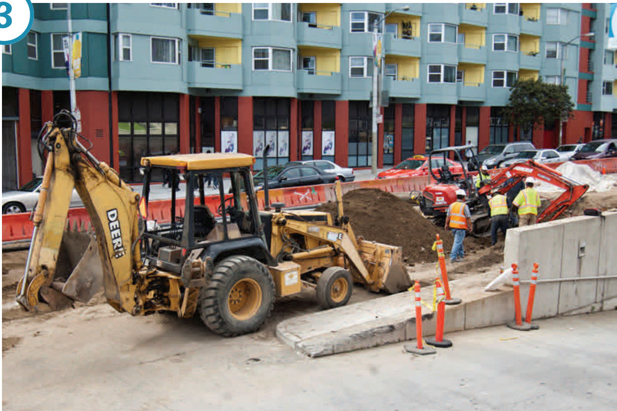
Headwall construction at the Yerba Buena/Moscone Station site has paused temporarily for workers to relocate a large-diameter water line.
