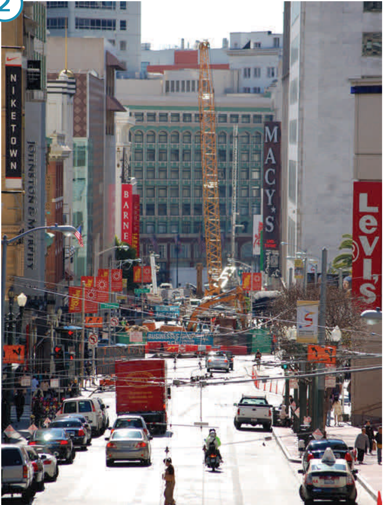
Looking south down Stockton Street from above the entrance to the Stockton Street Tunnel, toward the Union Square/Market Street construction site between Geary and Ellis, where station headwall construction is underway.
