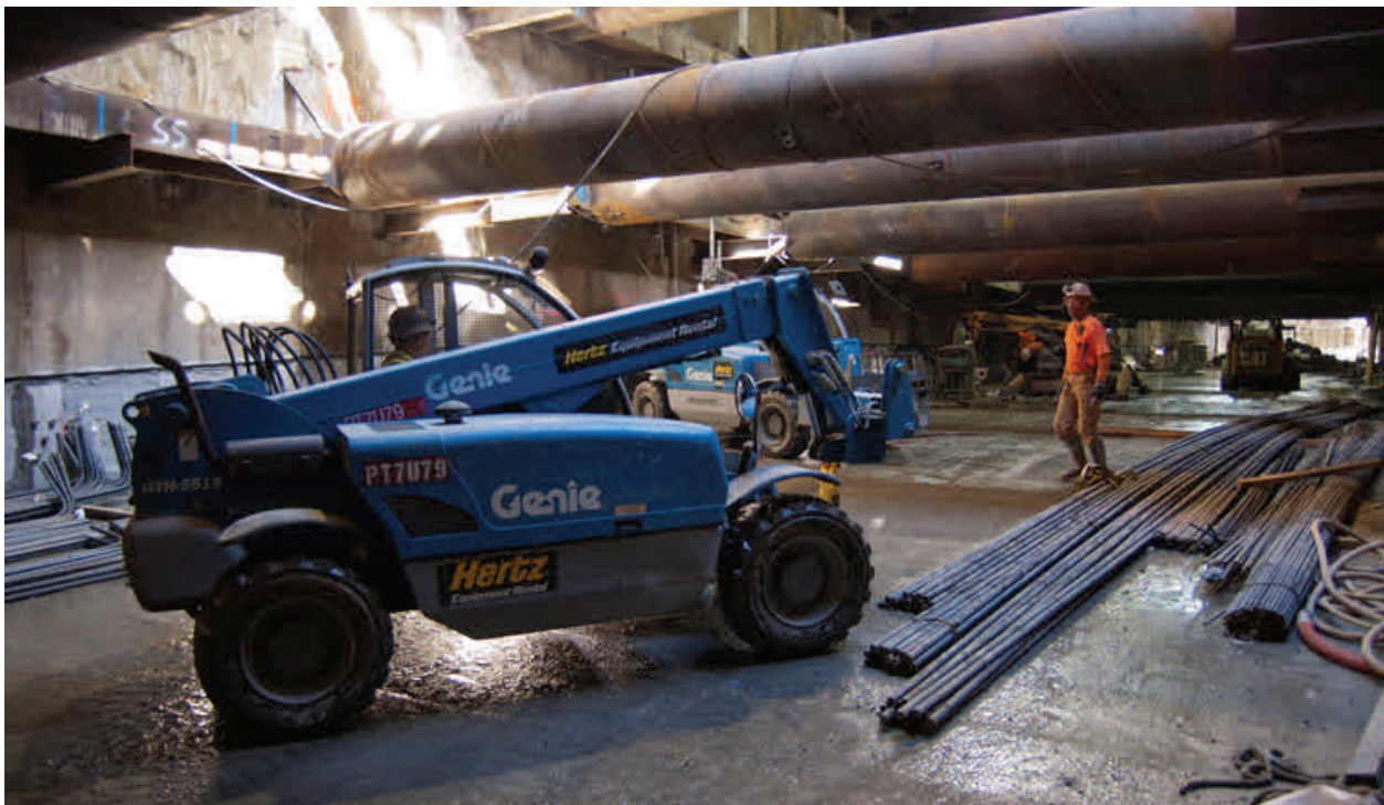
Crews have begun bringing in rebar that will be used to reinforce the floor slab of the launch box.
