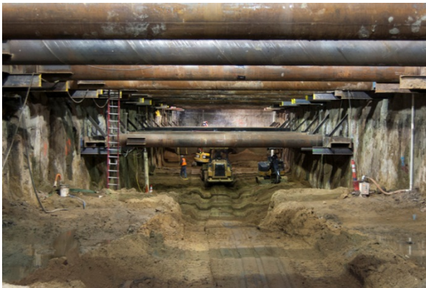
Inside Launch Box
