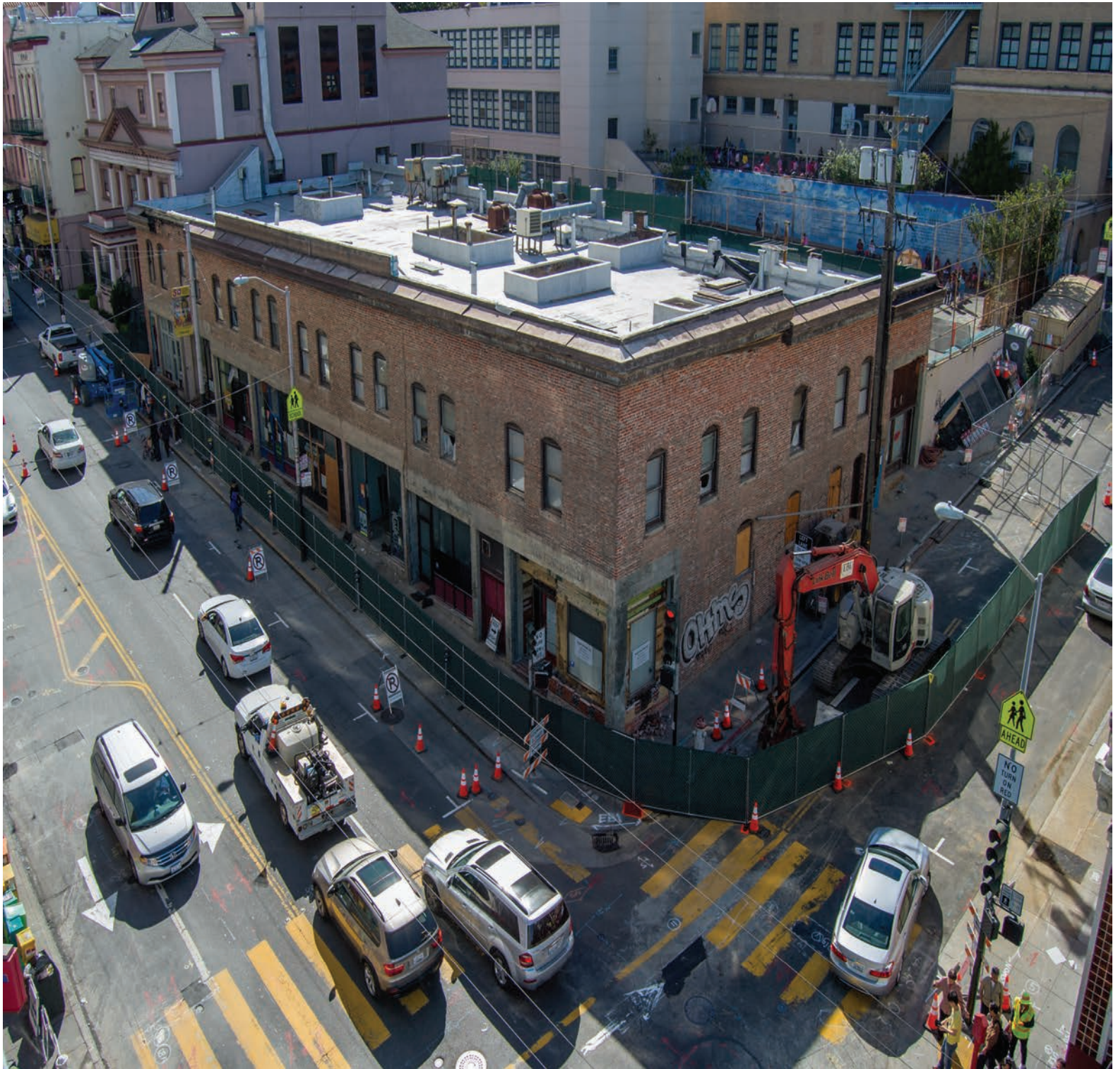
The original brick façade of 733-749 Stockton has been exposed, following hazardous material abatement. The building will be demolished to make way for the Chinatown station head house.
