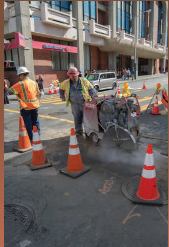
Potholing and utility relocation work has begun on Stockton at the future Chinatown station site. Workers can be seen here cutting the roadway prior to excavation.
