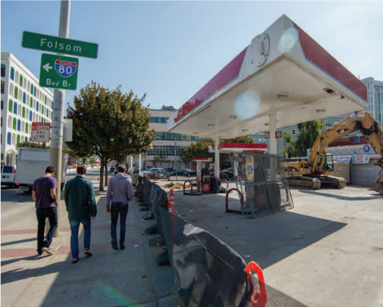
Demolition equipment arrived at the 76 gas station site in early October. The site has since been cleared to make way for the future Yerba Buena/Moscone station head house.
