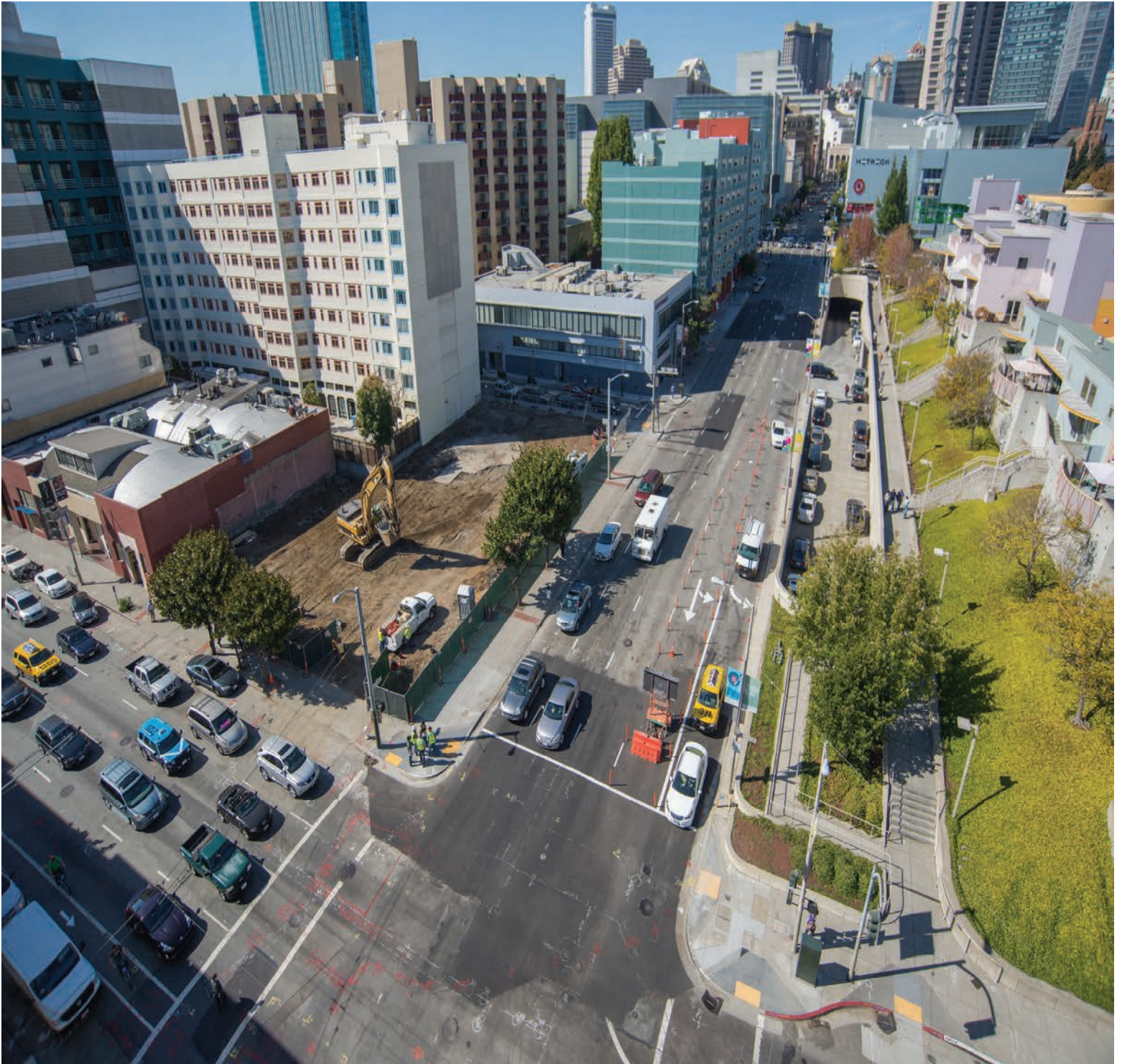
View looking at the intersection of 4th Street from the roof of 795 Folsom. Workers have demolished the above-ground structures of the former 76 gas station to make way for construction of the Yerba Buena/Moscone station head house.
