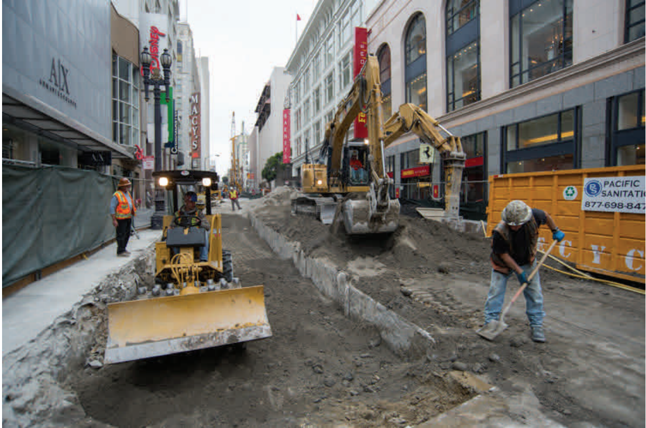
At the site of the future Union Square/Market Street station, crews are working to restore the work zone for traffic, ahead of the holiday moratorium which will go into effect before Thanksgiving.
