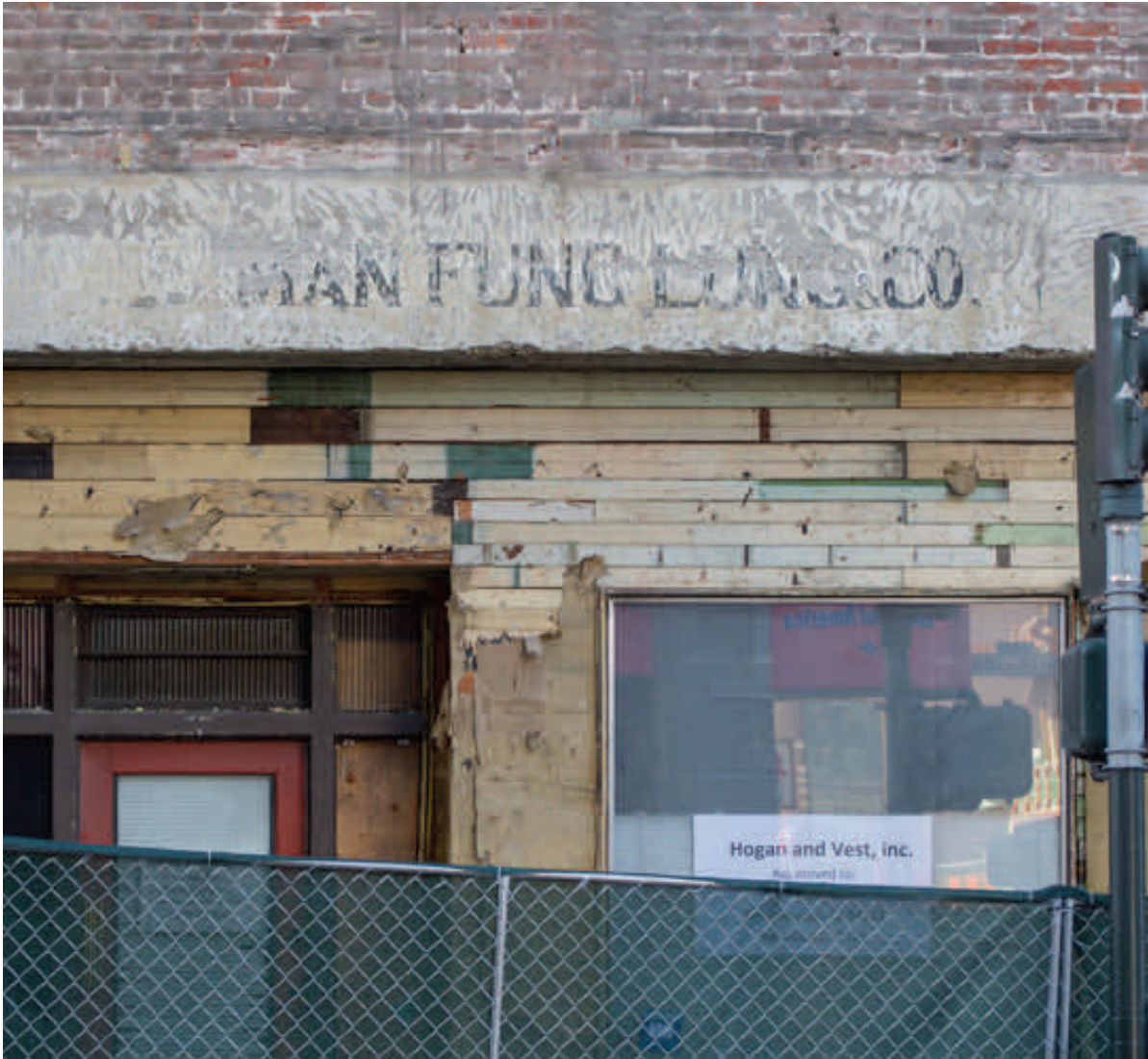
As part of hazardous materials abatement at the future Chinatown station site, the exterior stucco was removed prior to building demolition. Here, workers uncovered part of the sign of a former business.
