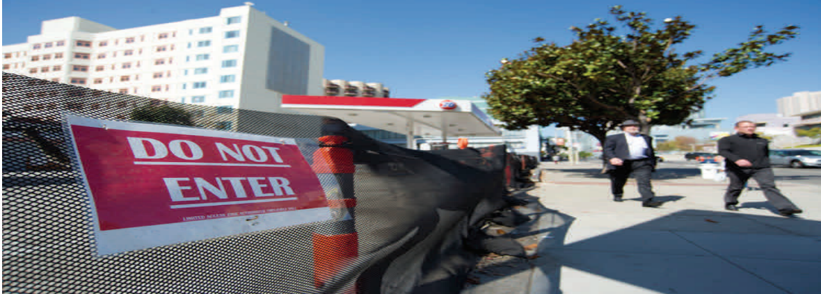
In October, 76 Gas Station was demolished to prepare the site for the future Yerba Buena/ Moscone Station construction.
