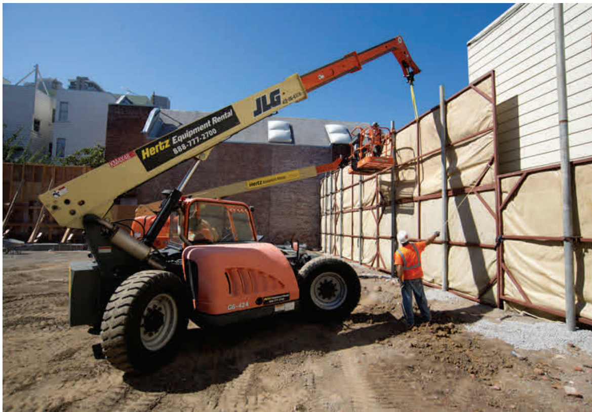
A temporary sound wall has been built at the site of the former Pagoda Theater in North Beach. Workers can be seen here lifting individual sections of the padded wall.
