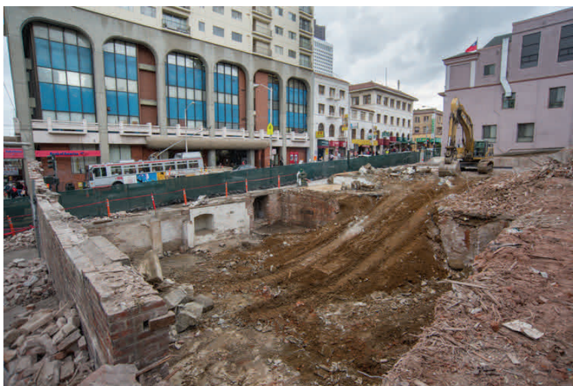
Demolition of the building at 933-949 Stockton commenced. The site will be used to build the head house for the future Chinatown Station.
