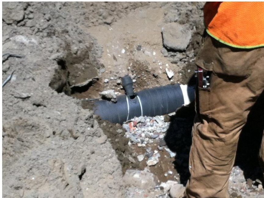
Dislodged nipple from the main pipe.
