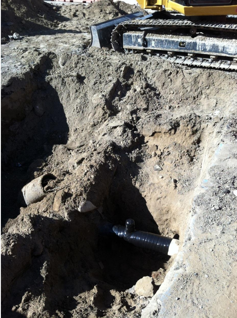
PG&E completed repair to the damaged gas line prior to it being backfilled.
